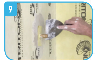
9 Use same trowel / mortar method to apply preformed collars at any plumbing exposures
