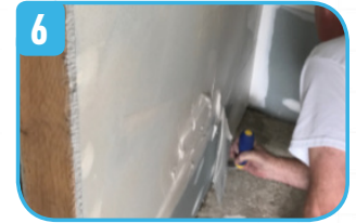
6 Skim coat wall where first WP™ sheet will go, then use 1/8" square notch (3mm) trowel to apply mortar bed
