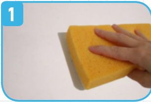
1 The substrate must be clean, even, and load bearing. Use a damp sponge to clean substrate.
